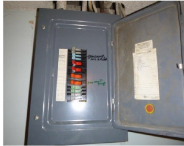
Recommend Zinsco sub-panel is replaced
