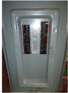
Recommend Stab-Lok panel is replaced
