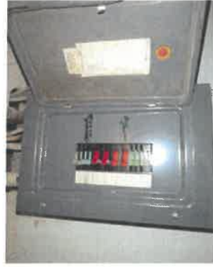
Recommend Zinsco sub-panel is replaced
