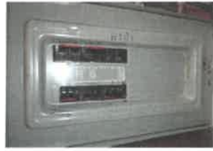
Recommend Stab-Lok panel is replaced
