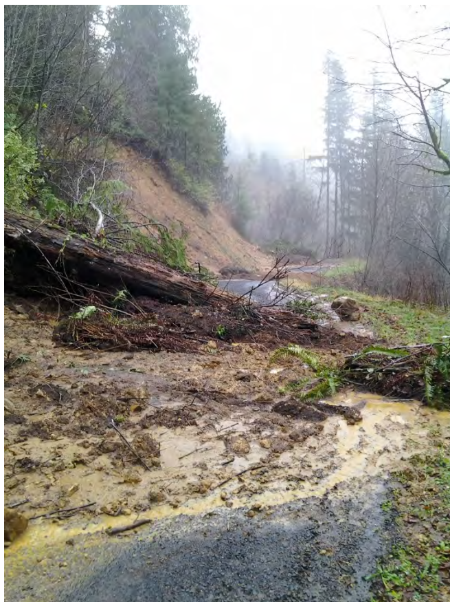
A landslide washes out a section of road near the Siuslaw River in 2014
