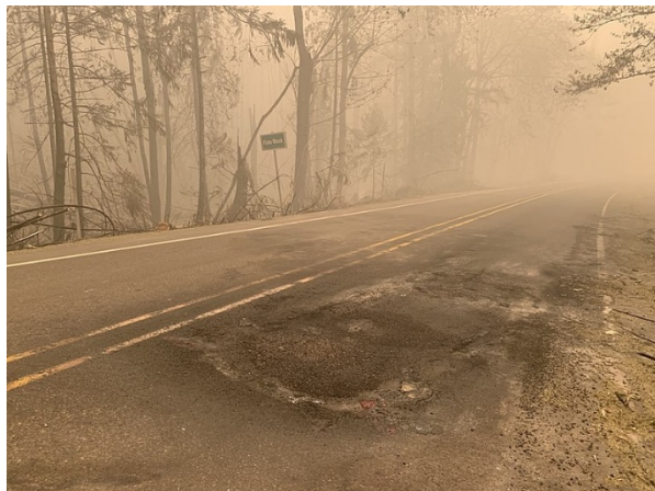
Damage along OR-126, McKenzie Highway during the Holiday Farm Fire (2020) | Source: Oregon Department of Transportation
